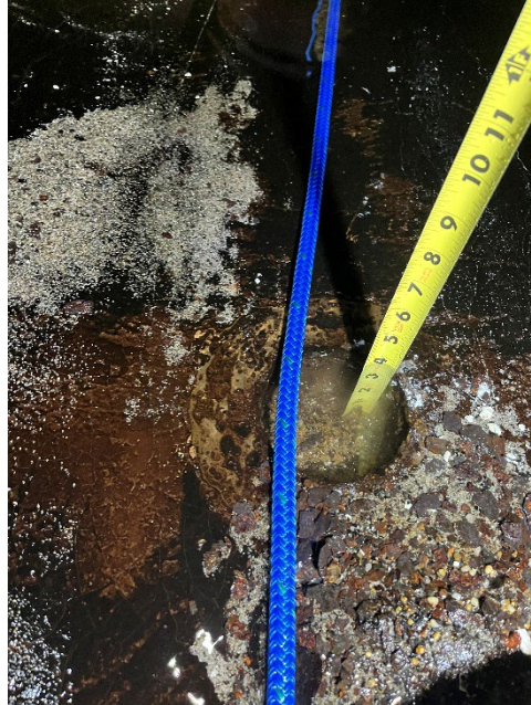
Figure 5: Observation #11 at Chemical Injectors
