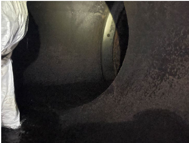
Figure 6: Observation #12B at Pipe Joint
