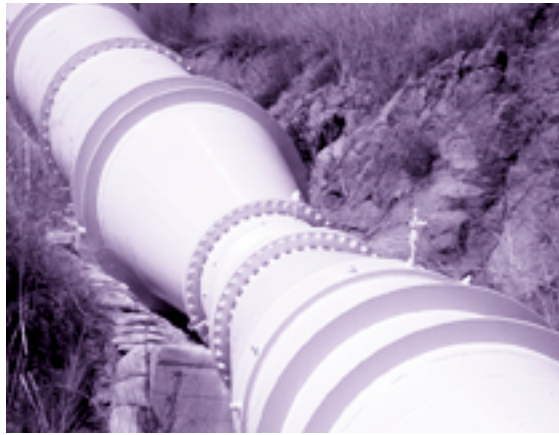
Pipe from Folsom Dam to San Juan Water Treatment Plant
