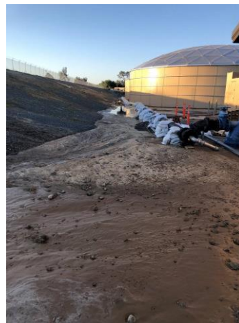
Figure 2 Eroded Embankment Material
