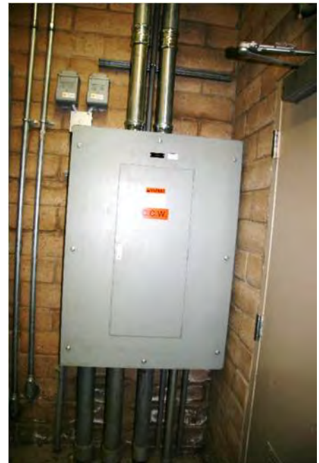
10/Panel Located Behind Door in Treatment Plant
