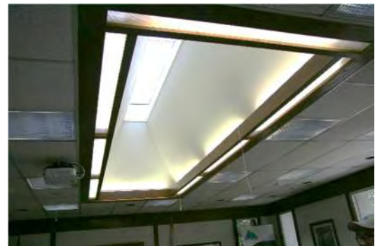
3/Lighting at Office
