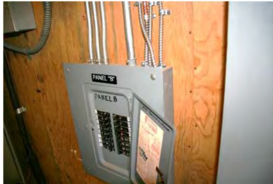
1/Sub-Panel at Office
