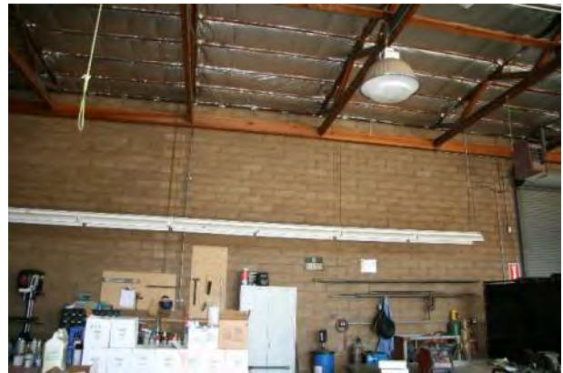
6/Lighting at Maintenance Building
