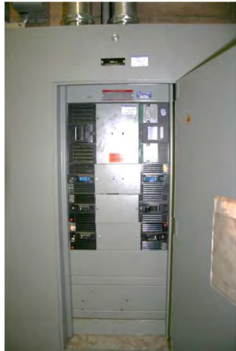
12/Panel Beyond Life Expectancy in Treatment Plant
