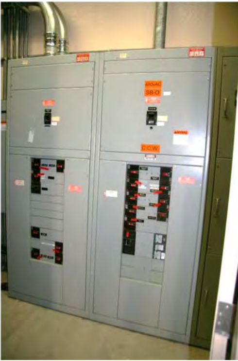
13/Switchboard Beyond Life Expectancy in Treatment Plant
