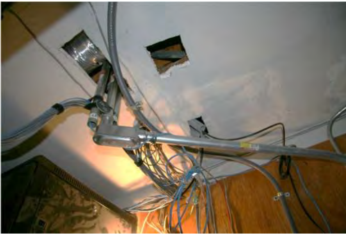
8/Ceiling of Low-Voltage Equipment Room
