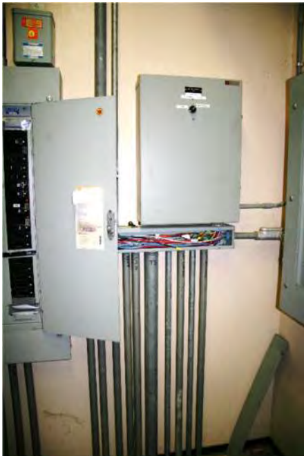
11/Code Violation in Treatment Plant
