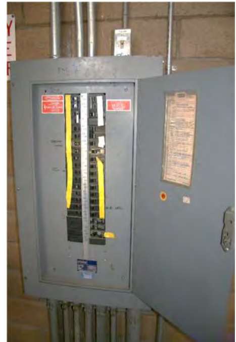
5/Sub-Panel at Maintenance Building
