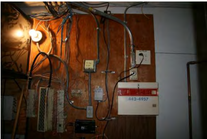
9/Backboard in Low-Voltage Equipment Room
