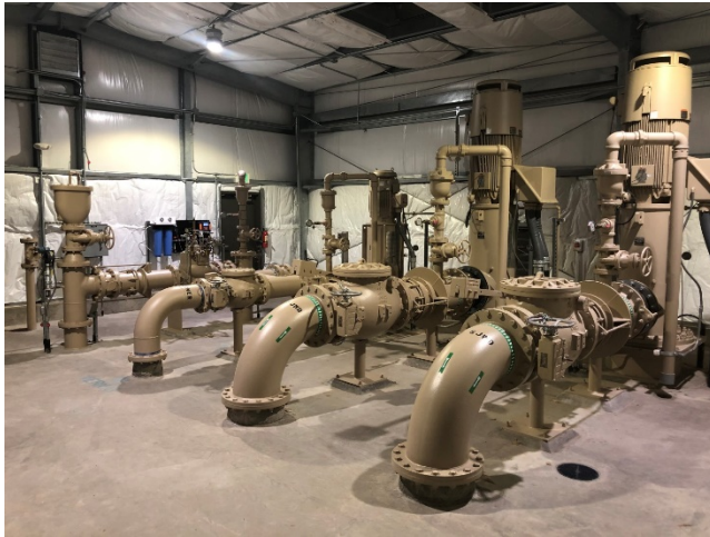
Figure 2: Antelope PRV Facility
