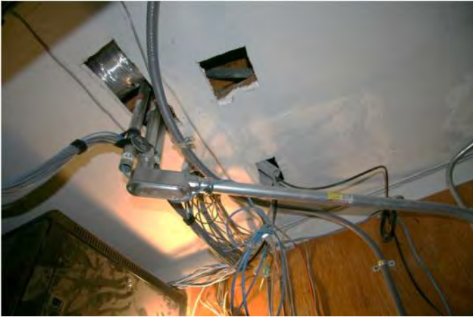
8/Ceiling of Low-Voltage Equipment Room
