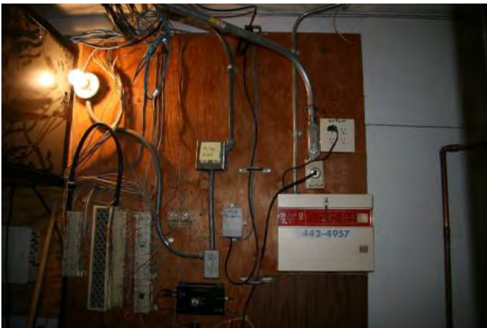
9/Backboard in Low-Voltage Equipment Room
