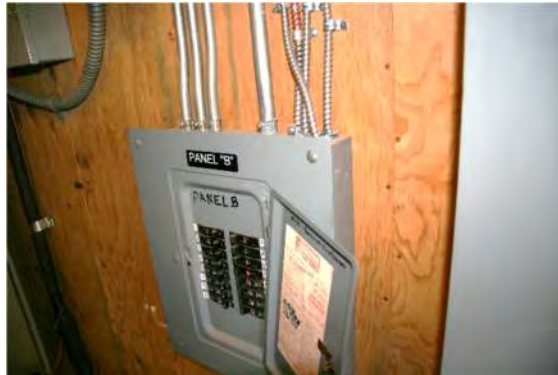
1/Sub-Panel at Office
