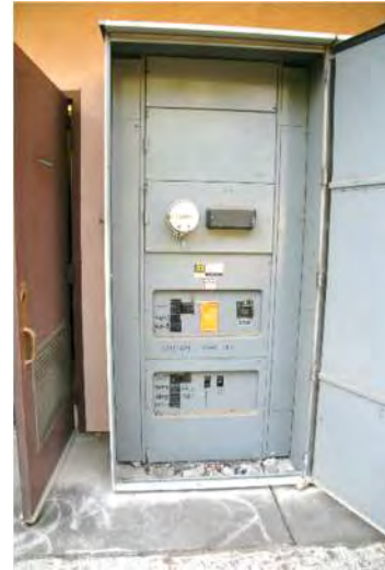
2/Main Switchboard at Office
