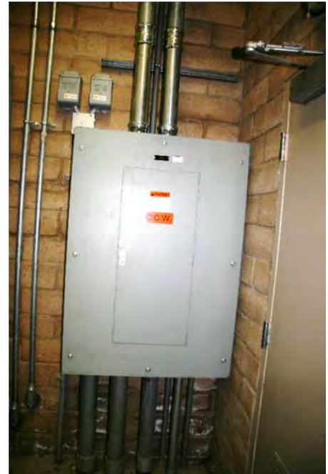
10/Panel Located Behind Door in Treatment Plant
