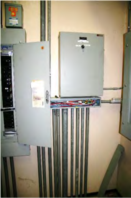
11/Code Violation in Treatment Plant
