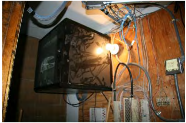
7/Backboard and IDF in Low-Voltage Equipment Room
