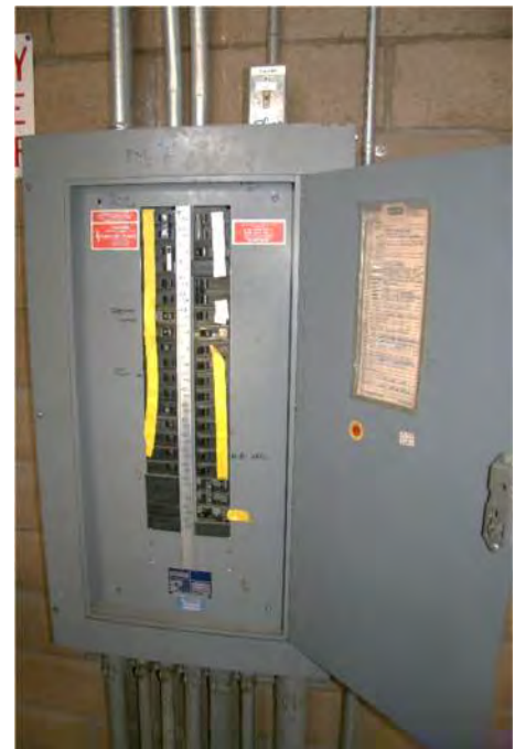
5/Sub-Panel at Maintenance Building
